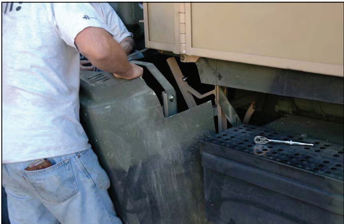
11.) Re-install original wheel well deflectors and ensure the wire from the side light has been connected. Note: fenders may need to be trimmed to make armor fit and will need to be trimmed to accommodate armor
